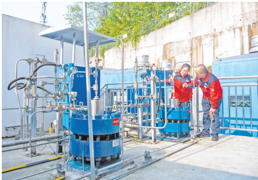
Workers conduct safety inspections in a hydrogen refueling station in southwest China's Chongqing. (PHOTO: XINHUA)
