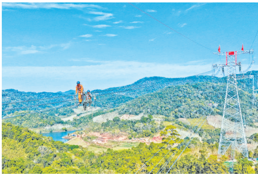
Engineers work on the transmission lines of the China-Laos 500-kilovolt interconnection project. (PHOTO: XINHUA)
