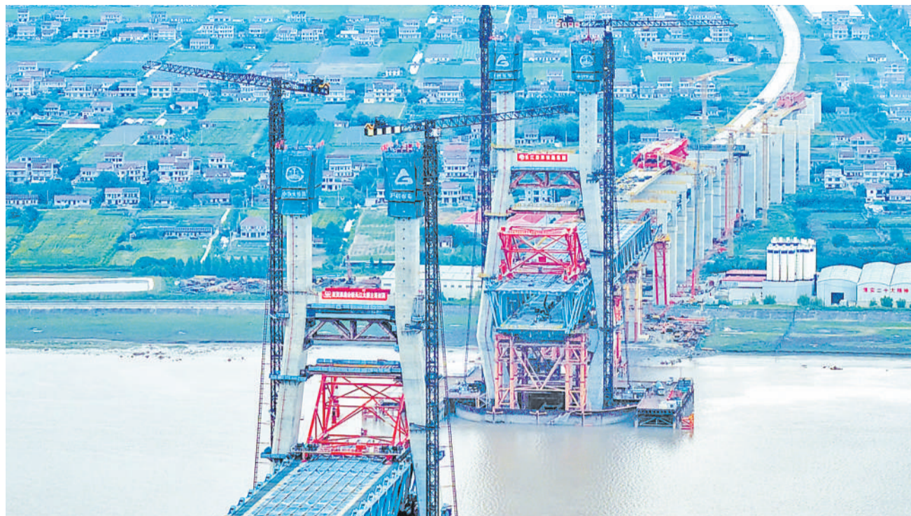
The No.3 and No.4 main pier caps of the Chongqi Highway and Railway Yangtze River Bridge are both topped out on September 29, 2025. (PHOTO: XINHUA)
