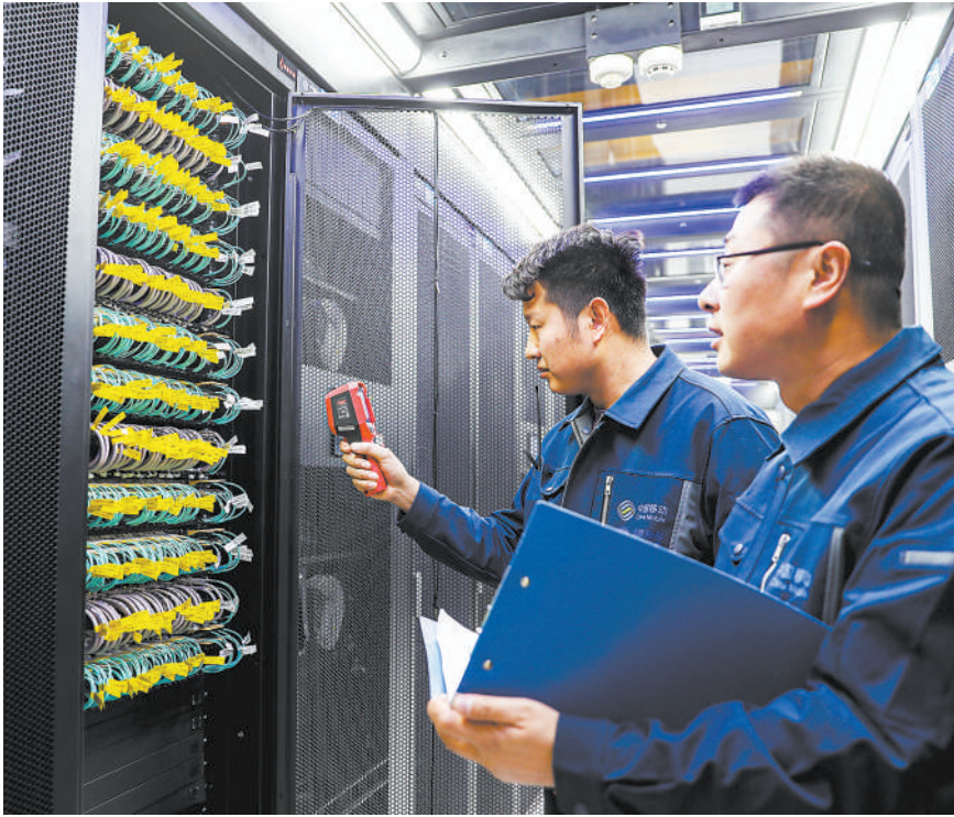
Engineers check equipment in a data center in Gansu province, January 6. (PHOTO: XINHUA)
