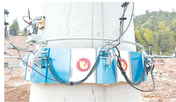
A climbing robot carries out safety inspection on the pier. (PHOTO: Jiangxi Consulting Investment Group)
