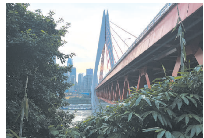
The Dongshui-men Bridge over the Yangtze River in Chongqing. (PHOTO: WANG Xiaolong)
