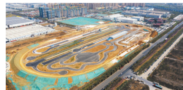
The R&D test site, located in the park of Volkswagen Anhui R & D center in Hefei, China's Anhui province, is under construction in March, 2023. (PHOTO: VCG)
