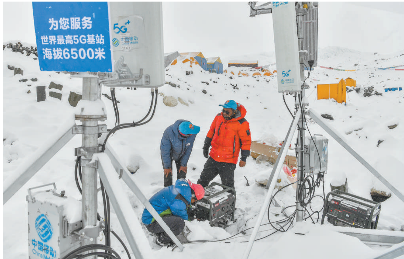
Staff members of China Mobile tested the signals of the 5G base station built at an altitude of 6,500 meters at the advanced base camp of Mount Qomolangma on May 21, 2021. (PHOTO: XINHUA)
