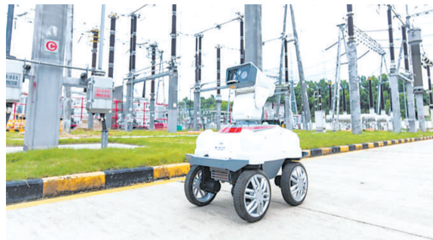
Shenzhen is using 5G robot technology for power grid monitoring and inspections. This has greatly improved efficiency compared to the past. (PHOTO: Science and Technology Daily)
