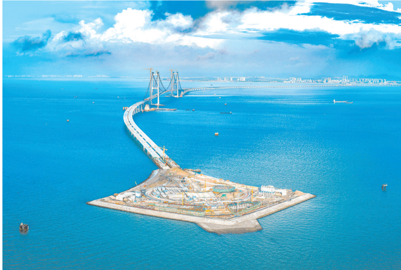
An aerial drone photo taken on June 20, 2023 shows the west artificial island of the Shenzhen-Zhongshan link under construction in south China's Guangdong Province. (PHOTO: XINHUA)
