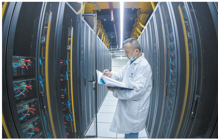
An engineer checks equipment at a Cloud Computing Big Data Center in Jiujiang city, Jiangxi province. (PHOTO: VCG)
