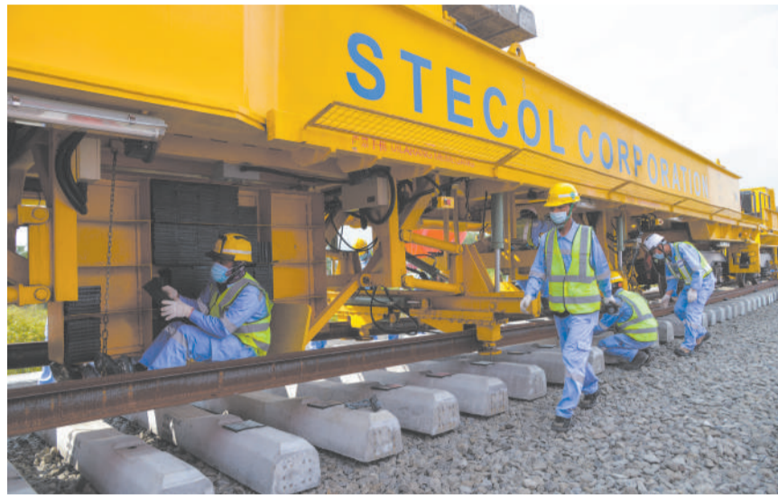
Workers at the construction site of the Jakarta-Bandung High-Speed Railway, designed with "China Standard" and will be furnished with equipment manufactured in China. (PHOTO: XINHUA)
