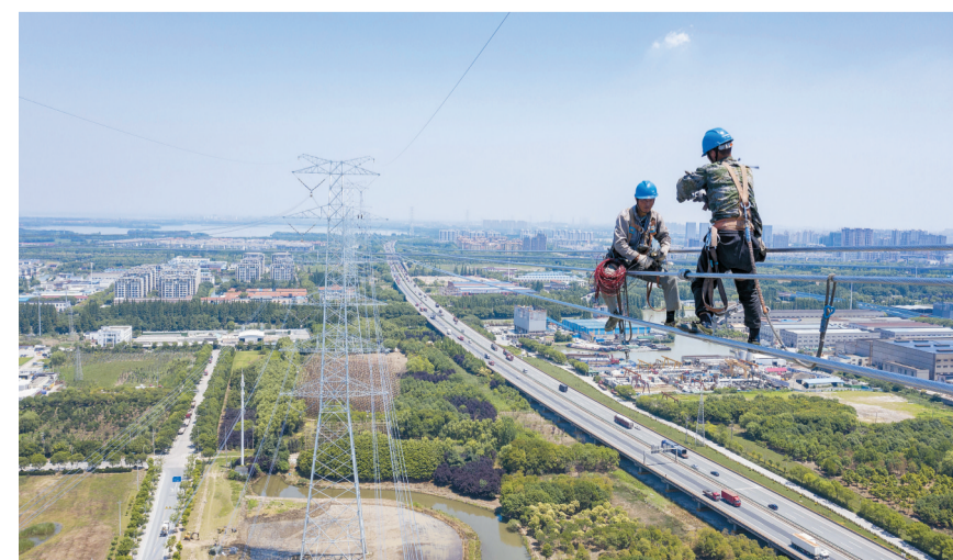
Workers set up wires for the transmission line in Kunshan city, east China's Jiangsu province. (PHOTO: VCG)
