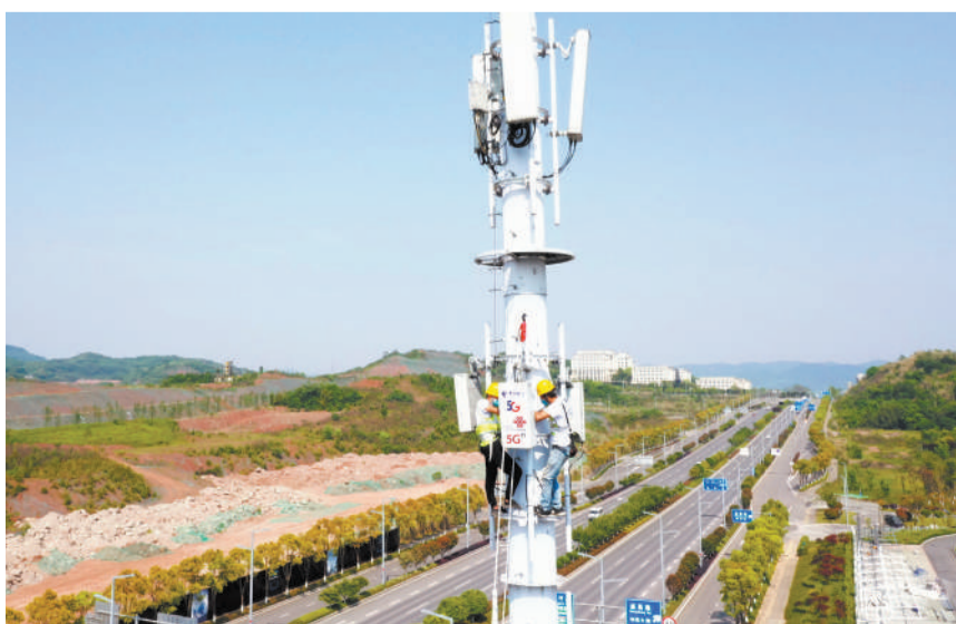
Technicians are working on a 5G base station in southwest China's Chongqing municipality. (PHOTO: XINHUA)
